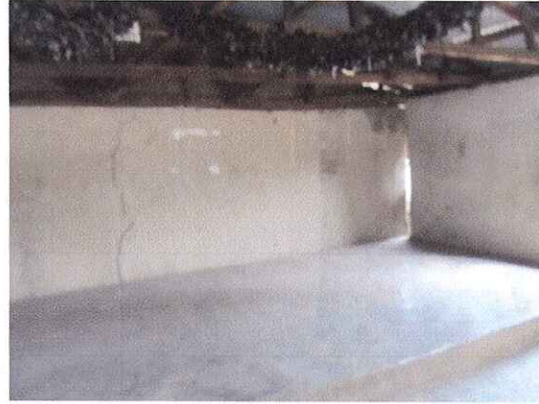
Bethel Baptist Church Wall cracked and separated from the other walls of the church
